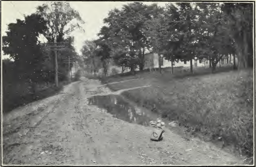
FIG. 1.—EARTH ROAD, SHOWING IMPERFECT DRAINAGE.
